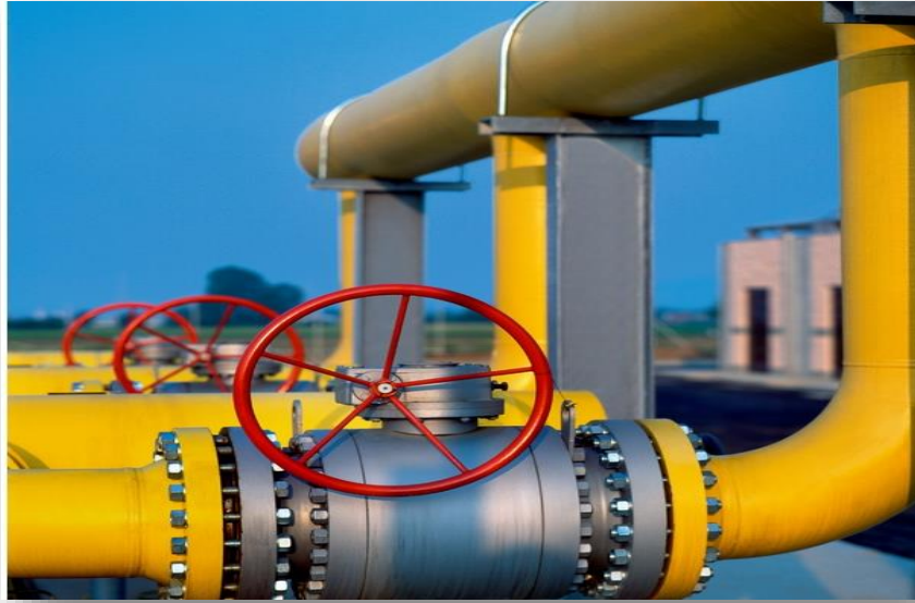
Figure 1.6 station de compression de gaz
