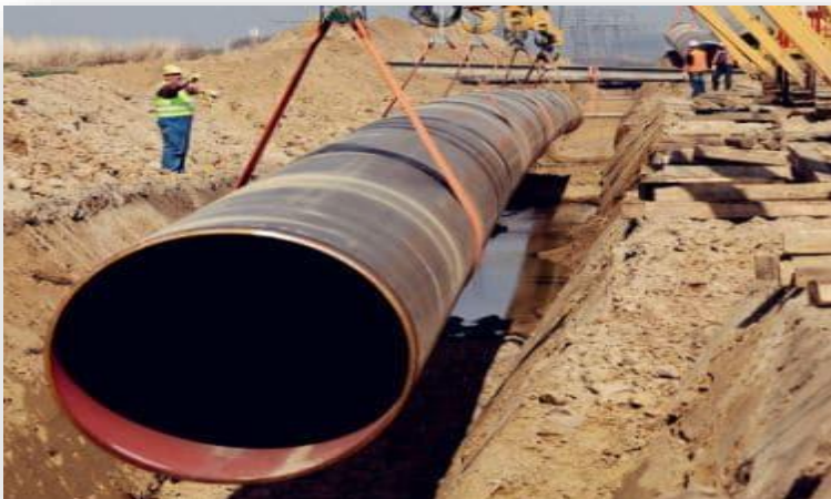
Figure 1.11 Pipeline en acier
