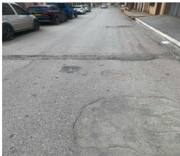
Fig II. 13: fissures importantes+ +usure
