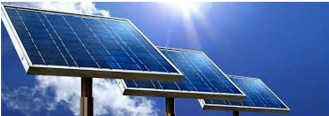
Figure III.6: Panneaux Solaires Photovoltaïques.[08]
