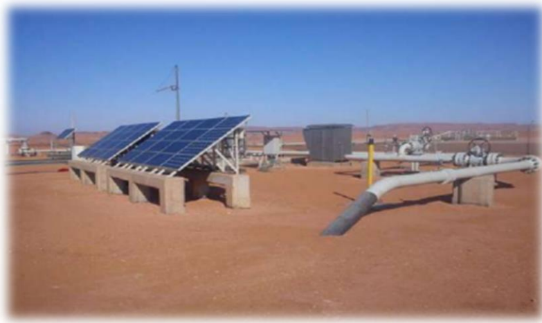
Figure (II.14) : Installation photovoltaïque.
