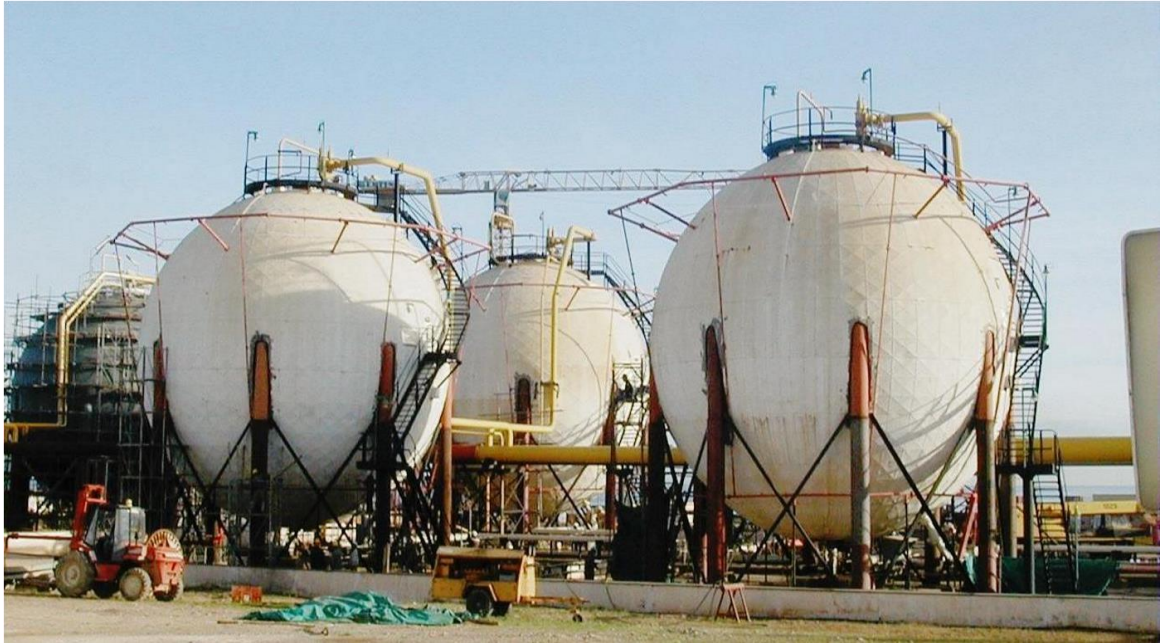
Figure 18: Sphères de stockage
