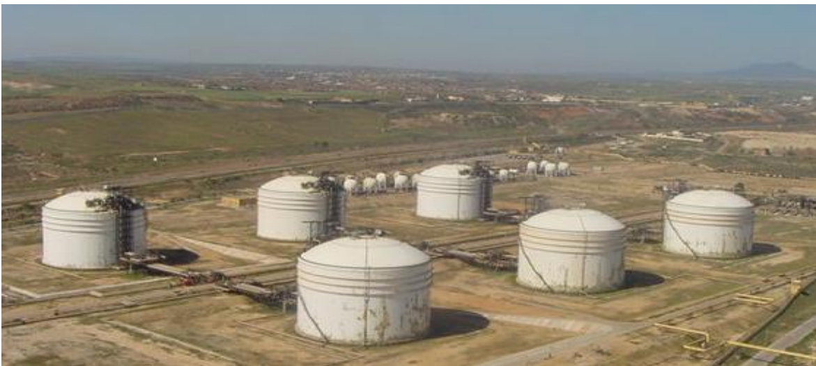
Figure 19: bacs de stockage
