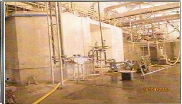
Figure III.6- cuve de stockage jus de sable.
