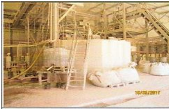
Figure III.7-cuve de stockage jus d'argile.
