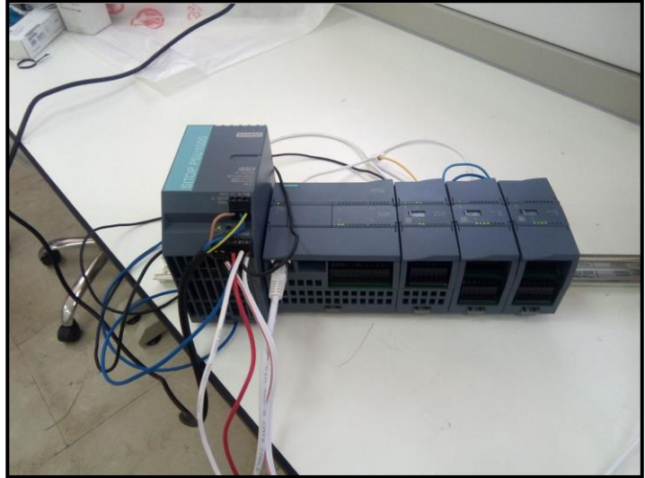
Figure XXXIXV.39 Project PLC Station.
