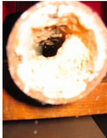
Figure V. 14 Conduite de fonte ductile
