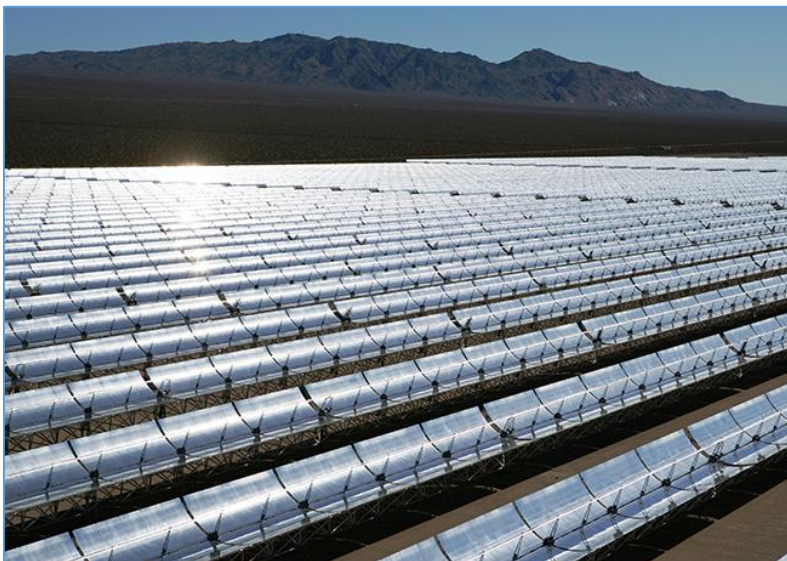
Figure 2.3 : Photo de la centrale CSP Nevada Solar One.
