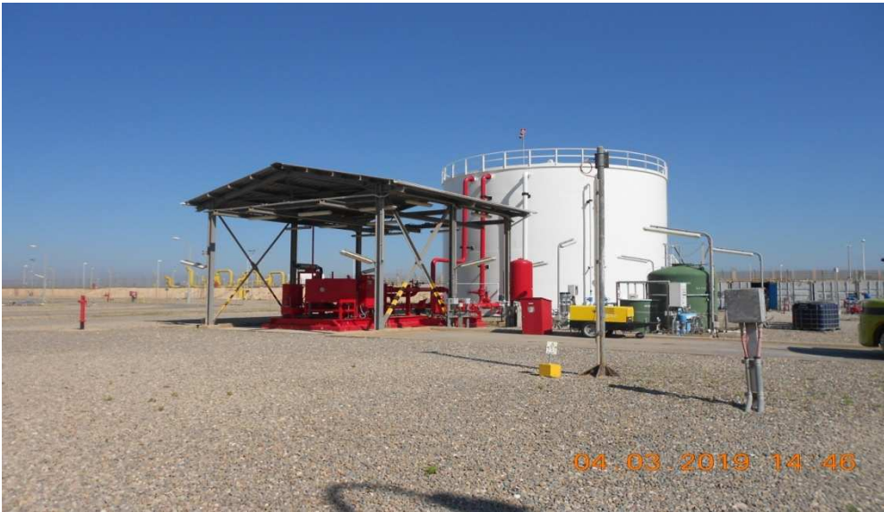
Figure IV-6 Station anti incendie
