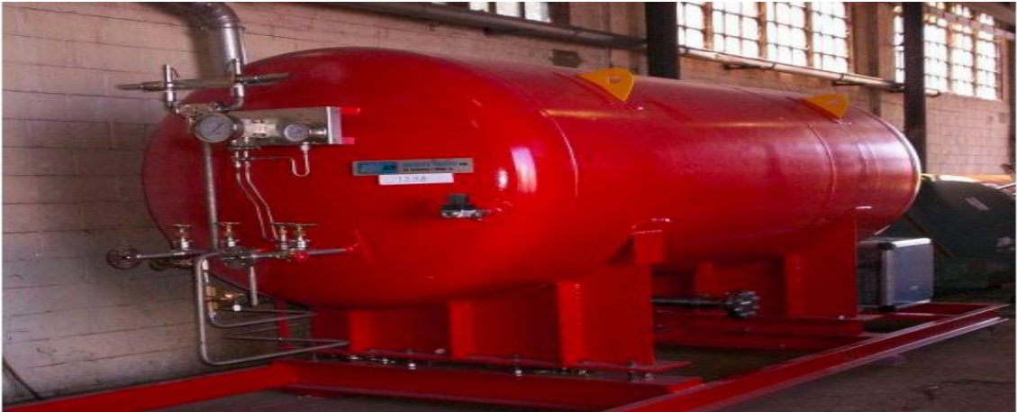
Figure 3.8: CO2 fire extinguishing.[3]
