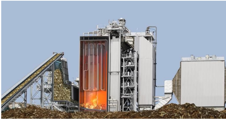
Figure 32: La centrale Biomasse
