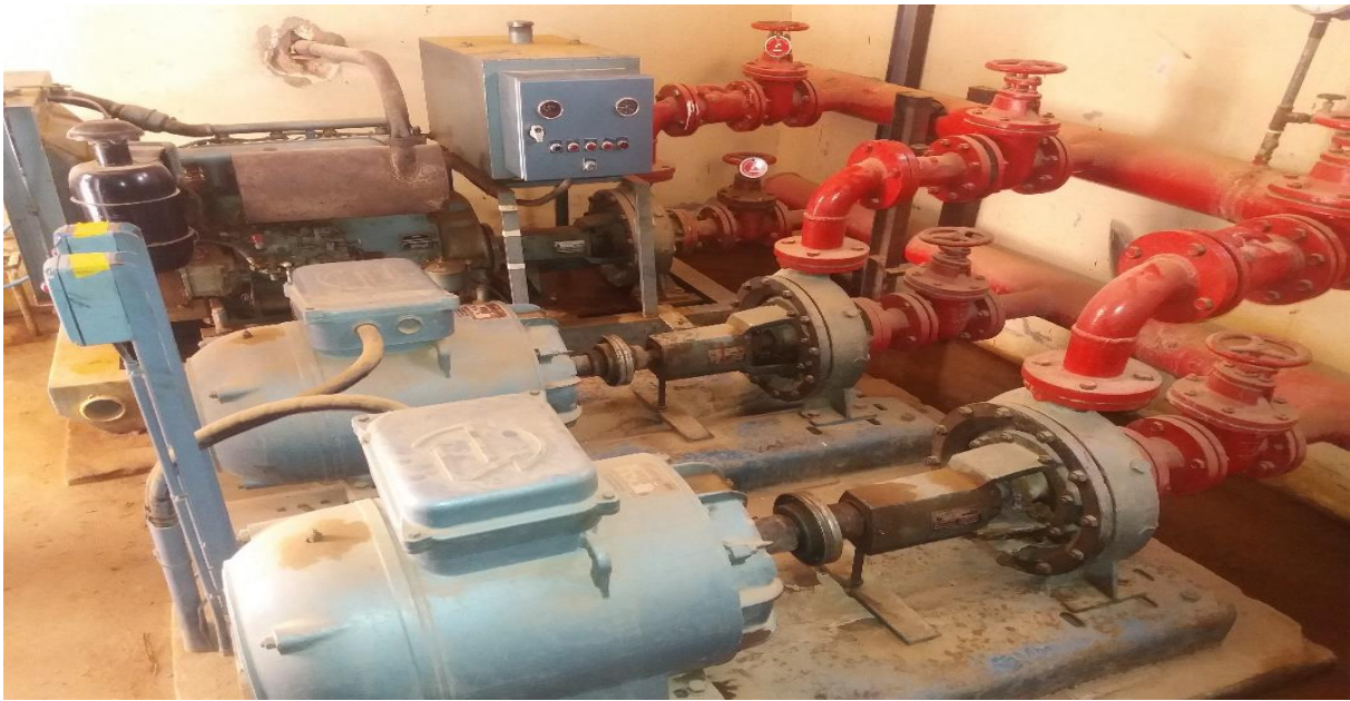
Figure III.1 : Locale des pompes
