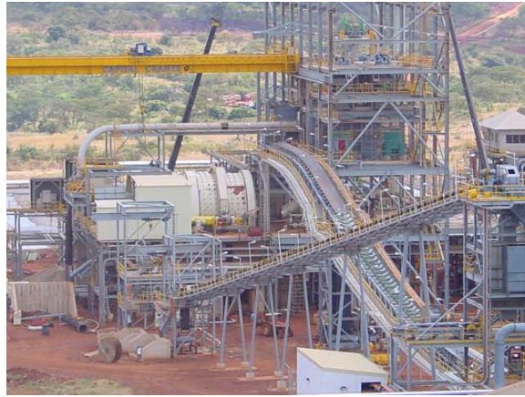
Figure32: SAG MILL (Source: processing department, TMLSA)
