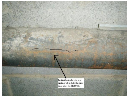
Figure (I-14) : Fissuration des pipelines
