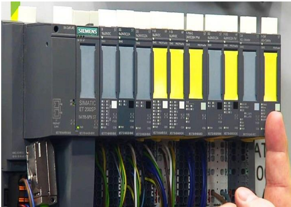
Figure06: automate programmable industriel
