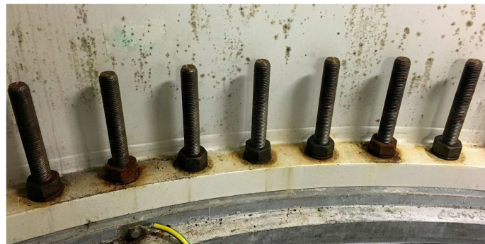
Figure II.4: Wind turbine anchor bolts (foundation bolts) affected by corrosion and Mold. [41]
