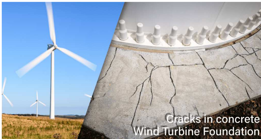
Figure II.3: Turbine failure due to weak foundation. [40]
