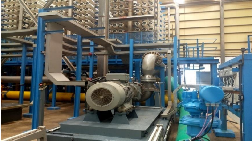
Figure II. 12: la pompe Booster
