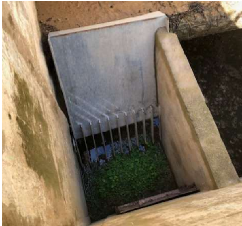
Figure II.5 : La grille grossière de la station de relevage.
