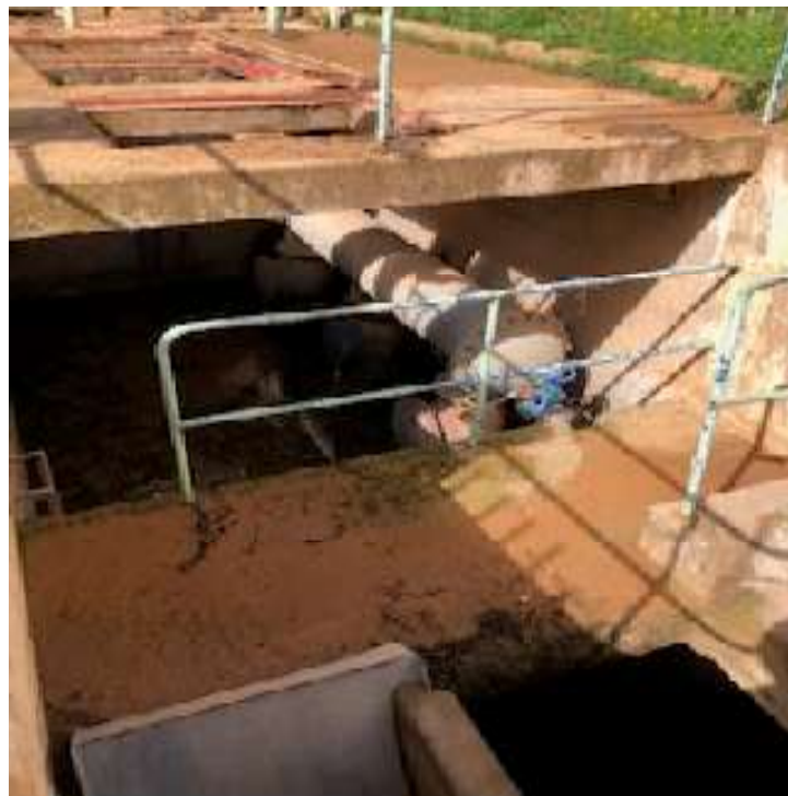
Figure II.4 : Station de relevage.
