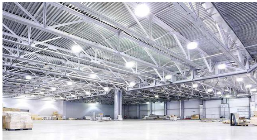
Figure 1.5: Example of lighting for industry
