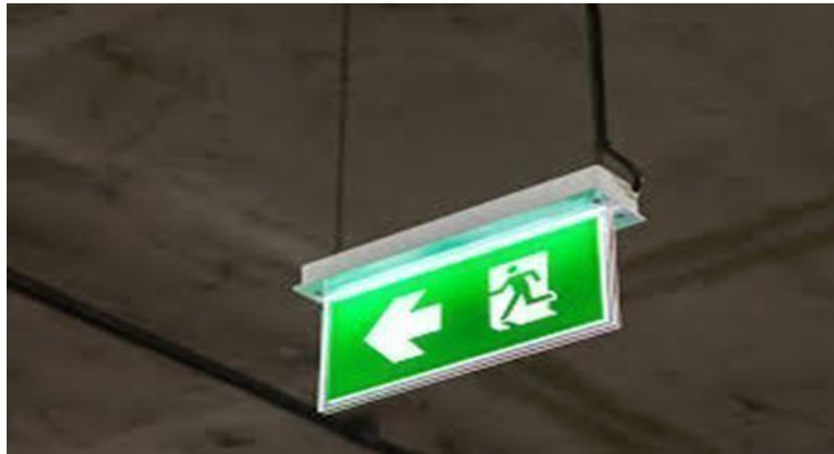
Figure 1.7: Example of lighting in the field of security
