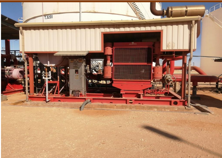
Figure 4.5 Pompe diesel P3201C
