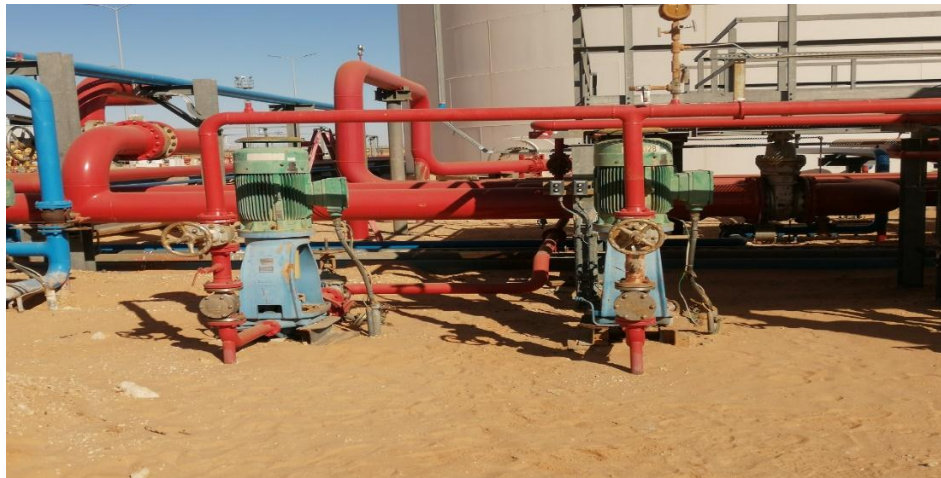
Figure 4.3 Pompes jockey P3202A/B
