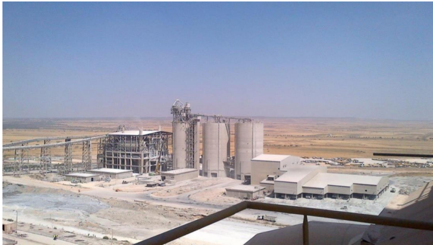
Figure 18: Silos de stockage
