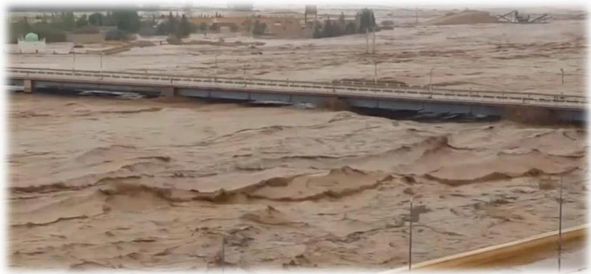
Figure 21: The Sidi Hakoum Bridge moments before it collapsed during the 2016 floods
