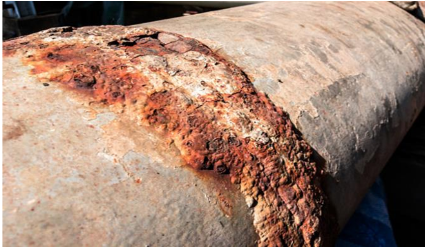
Figure 1.2-Corrosion externe de pipeline
