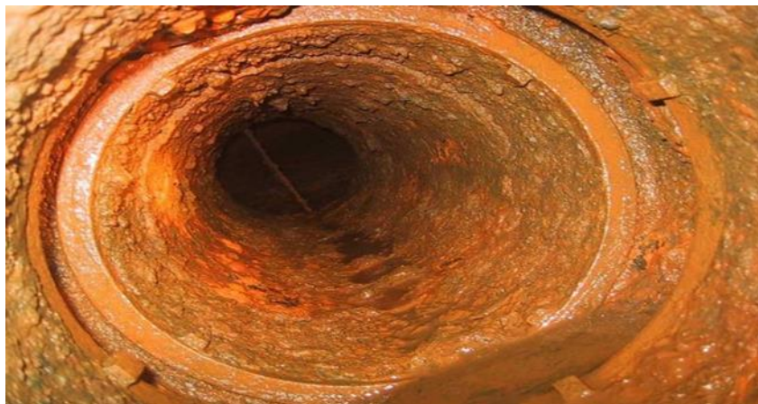
Figure 1.3-Corrosion interne de pipeline
